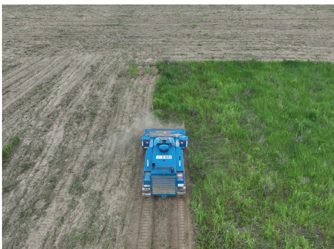
Specialised machines are used to prepare the ground, accelerating the work of deminers. (Ukraine, 2024)
