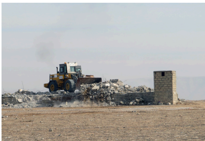
Armoured construction engines are used to clear rubble from partially destroyed buildings. (Iraq, 2021)
